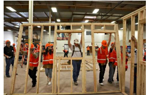
ACE students led by a carpenter journeyman, erecting a frame they just built.
